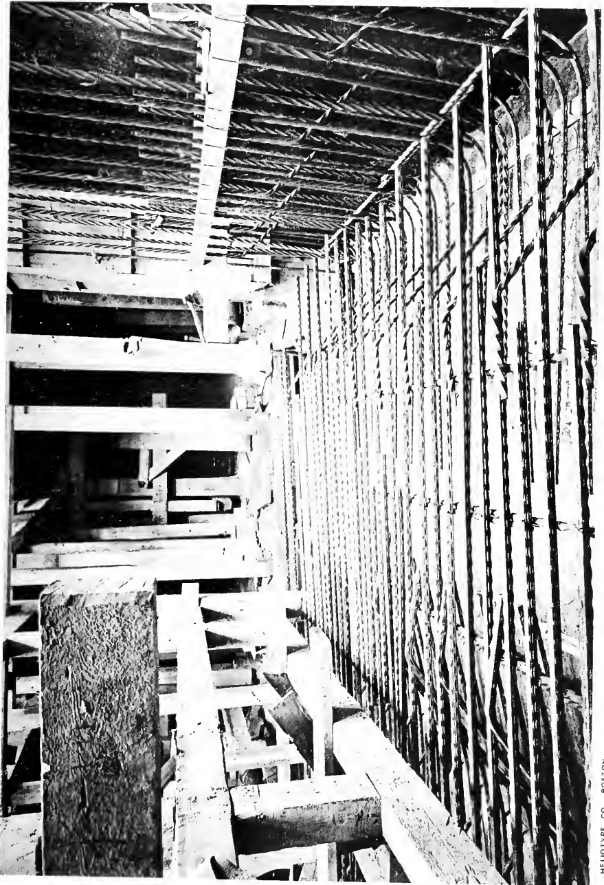
BOYLSTON STREET SUBWAY, SECTION 4. STEEL RODS PLACED FOR INVERT REINFORCEMENT ABOUT 50 FEET WEST OF TOWER OF OLD SOUTH CHURCH.
